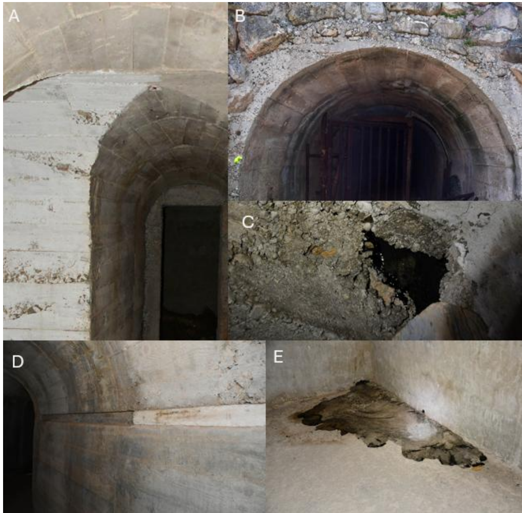
Figure 8: A: Timber formwork impressions preserved in the tunnel walls; B: Entrance arch and external stone work of the main entrance; C: Tar sheeting visible above a door frame; D: Channel in wall which still contains a wooden beam; E: Tar seep on the floor.
